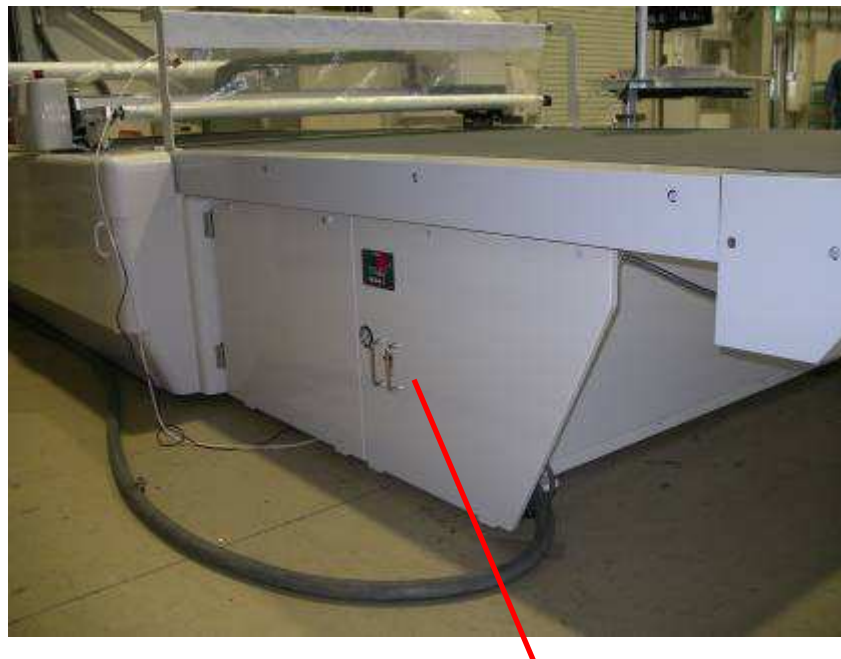
Main power supply switch
